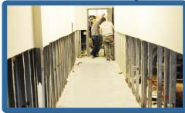
After Hurricane Sandy, workers remove water damaged sheet rock to prevent mold growth. Photo by George Armstrong/FEMA
